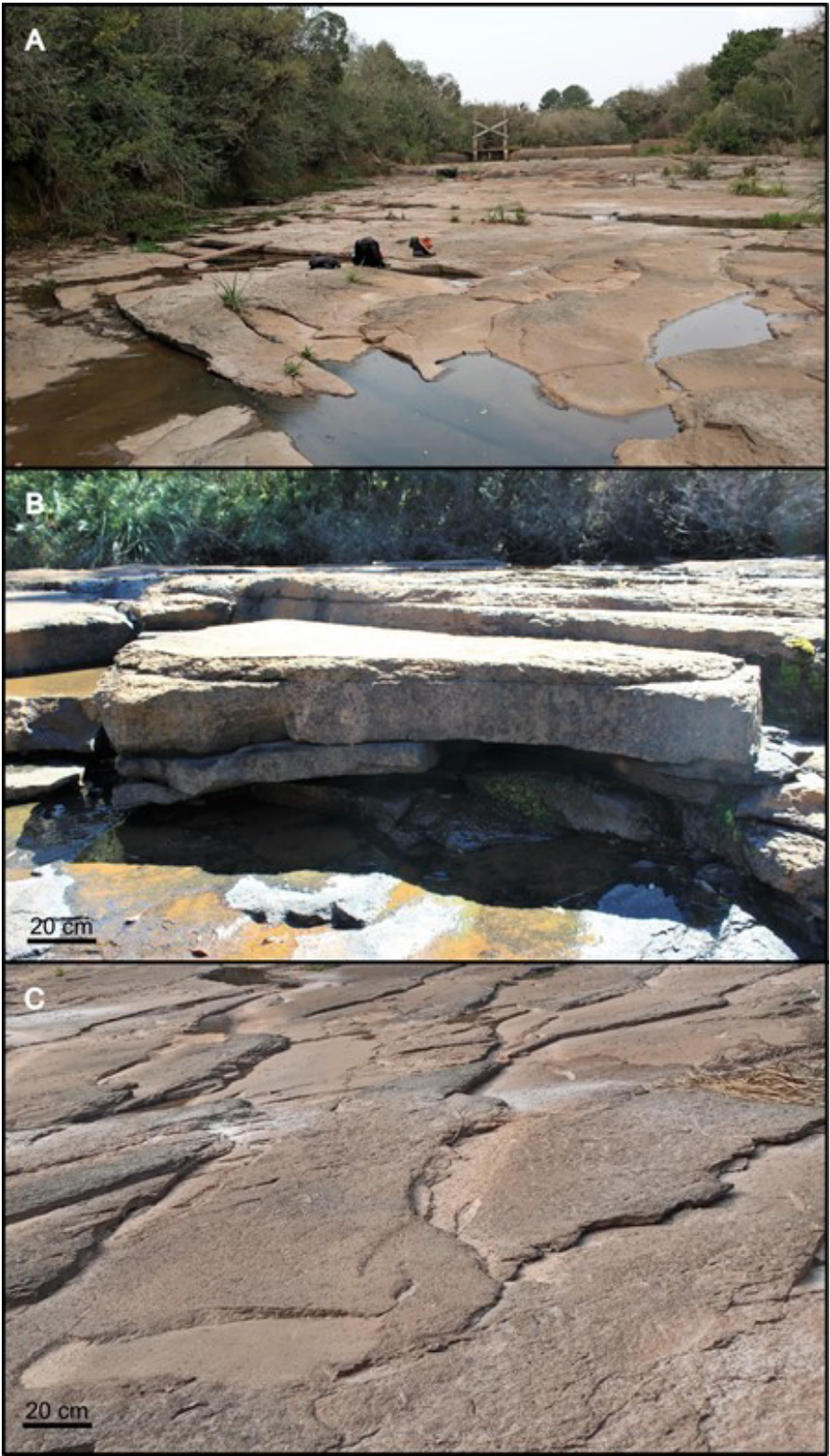
Figure 3 Fractures present in the study area: A. Set of vertical joints, visible on the right side of the channel; B. Horizontal joints located downstream of section; C. Sub-horizontal joints located on the left side of the section.
