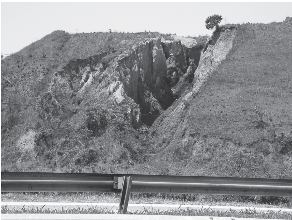
Figure 9 - Deep gully along the state road RJ-122 in the municipality of Cachoeiras de Macacu
