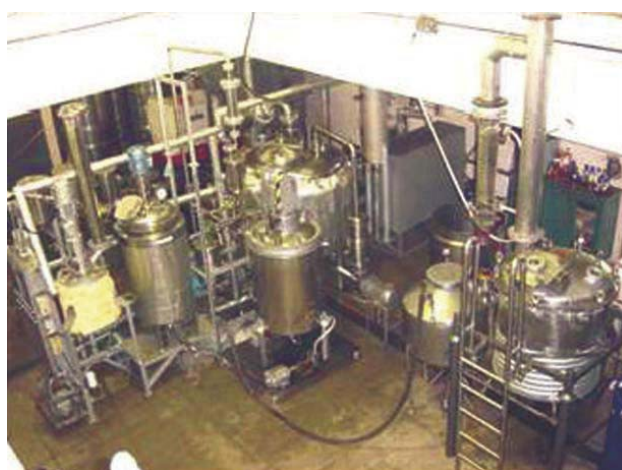
Figure 12 – Biodiesel plant of the IVIG- Coppe-UFRJ (Project of electricity generation from palm oil in Pará).
