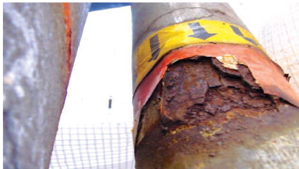
Figure 2: A pipe with local corrosion damage.
