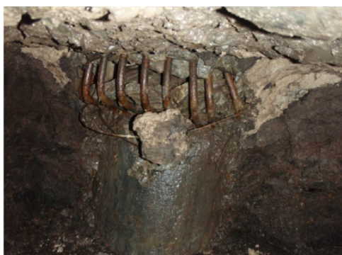
Figure 2 Bridge pile foundation damaged at the upper end due to the lateral movement of the soft clay deposit
