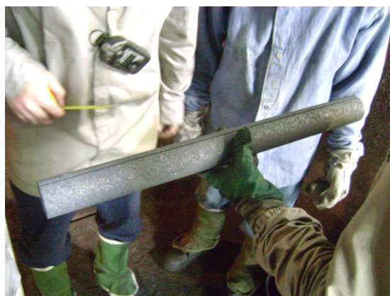
Figure 3. New refractory cylinder to restore the sample hole into the refractory lining.
