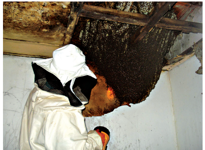
FIGURE 2 - Africanized honeybee swarm under the roof of a building.
