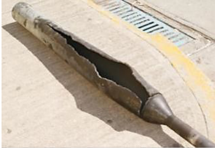
Figure 1. Perspective view of the section of tube failed.
