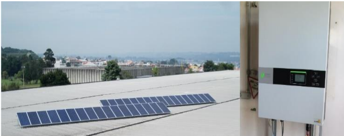
Figure 1 – Grid-Connected Photovoltaic System and Inverter of UTFPR – Curitiba
