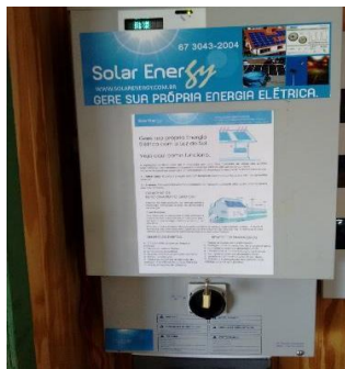
Figure 3 - Inverter of the UTFPR GO central campus. Source: Authors
