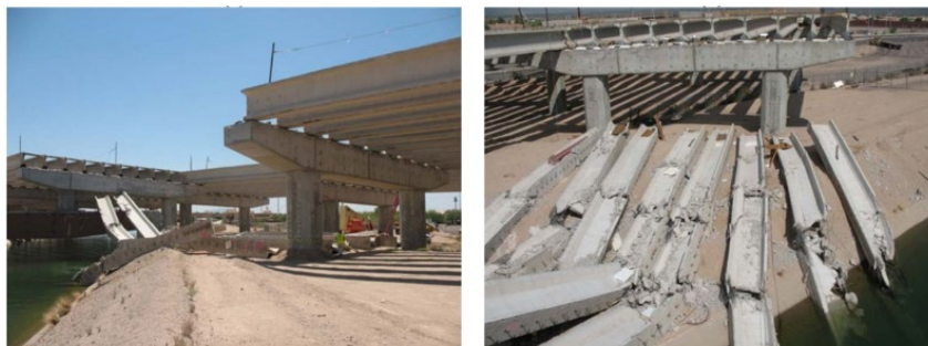
Figure 1. Beam collapse in Arizona (EUA). Source: Oesterle et al. [4]
