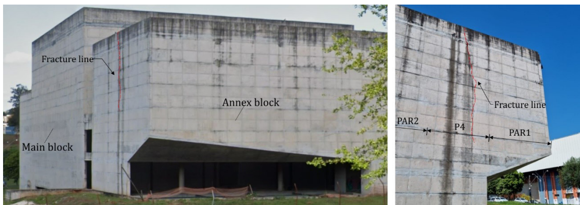
Figure 1. Reinforced concrete building with a localized failure.
