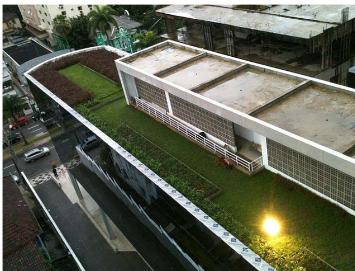
Figure 22. Green roof of the Ana Costa building, in Santos, SP. Source: NM Inovações (2020)
