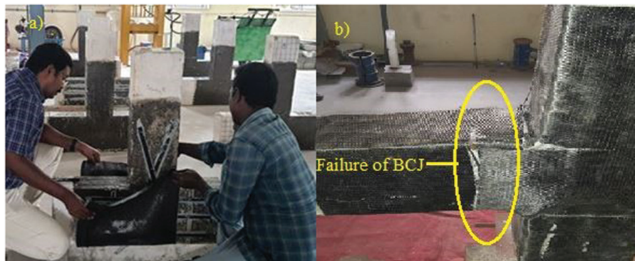
Figure 8: a) Applications of CFRP b) Failure mode of beam column joint.
