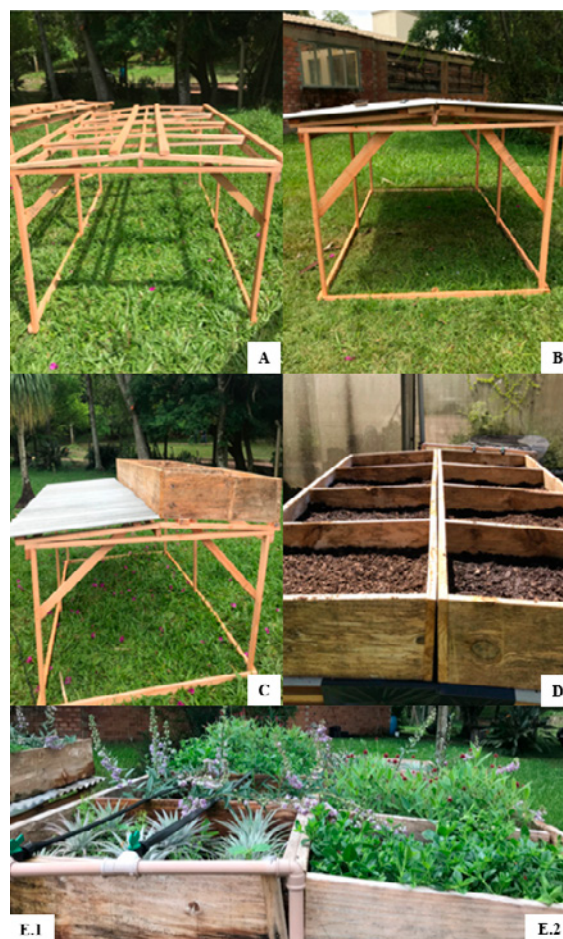
Fig. 2. Illustrations of the prototype built to receive the next layers of the green roof system are shown and after installation. In (A), the base of the structure is depicted; in (B), the base is shown after receiving the fiber cement tile; in (C), the prototype with a box is illustrated; in (D), the prototype is depicted already installed and filled with pine bark substrate; in (E), one of the blocks with developed plants is shown. Subsequently, (E.1) shows the drip irrigation system, and (E.2) shows the block without an irrigation system.
