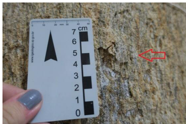
Figure 4. Millimeter-order blistering indicated by the red arrow.
