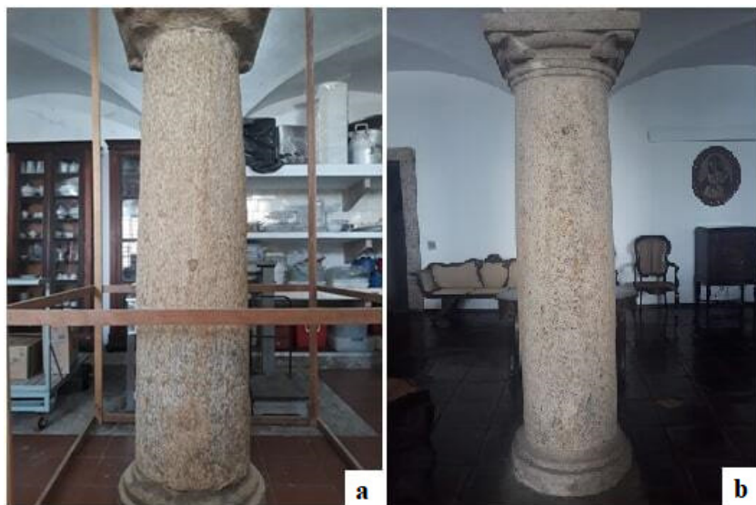
Figure 1. a: Column with accelerated alteration located in the deposit. b: More intact column located in the cloister.
