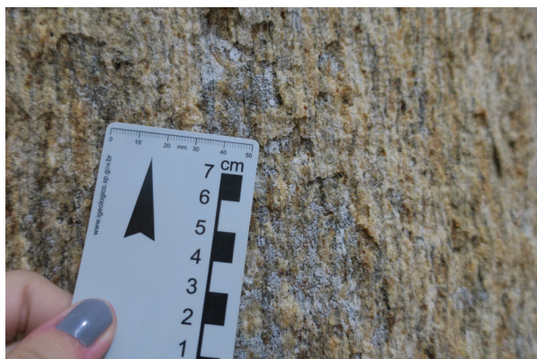
Figure 3. Occurrence of efflorescence. Accumulation of poorly coherent salt crystals on the gneiss surface.
