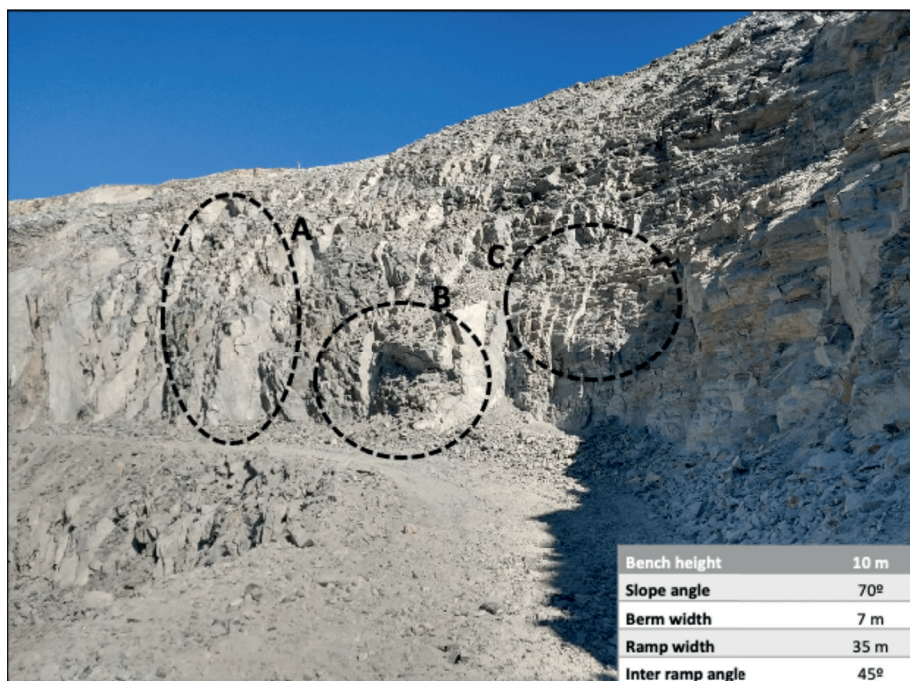
Figure 1. Slope conditions at the mine site and geometrical parameters according to mining staff. A shows geometry issues, B big blocks formed by excessive blast damage and C crest loss.
