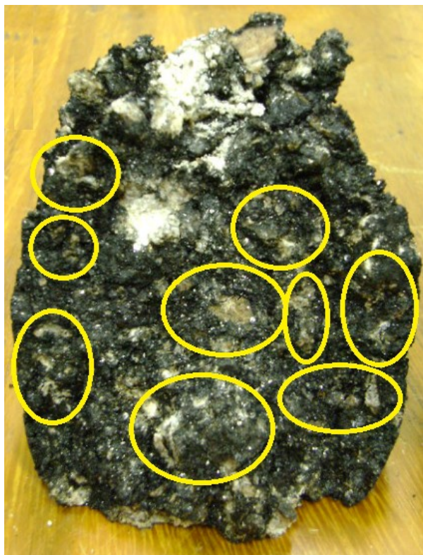
Figure 8. Removal of the asphalt binder coating due to deleterious action of water.
