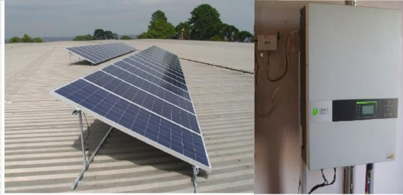
Figure 3: Neoville headquarters' Photovoltaic Panel 9 .
