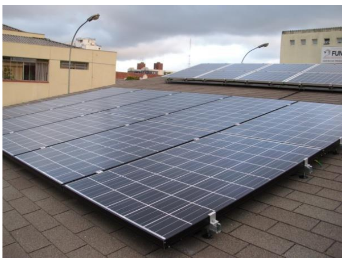
Figure 2: GO's Photovoltaic Panel 7 .
