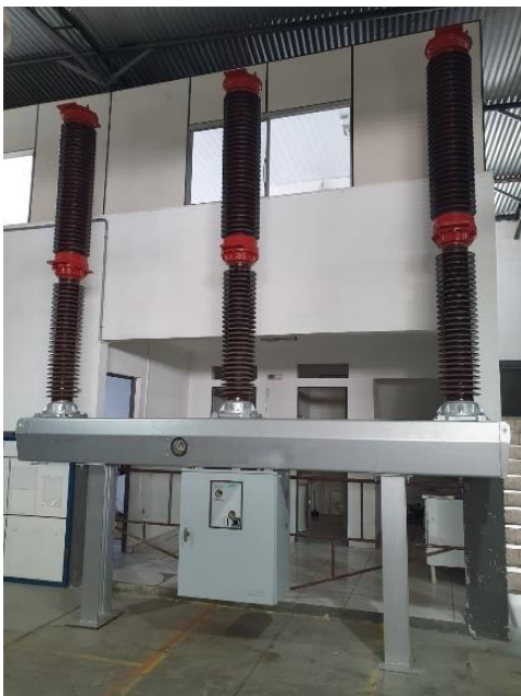
Figure 2. Circuit Breaker Testing Laboratory.
