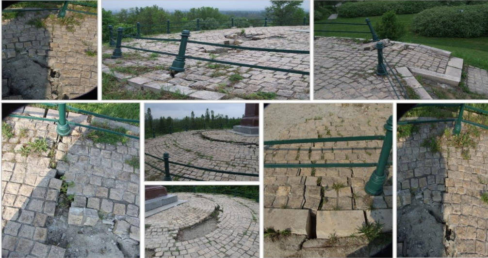
Figure 4: The view of destruction of the upper view balustrade of the Wanda Mound in 2010 and 2012, as a result of intensive and long term precipitation
