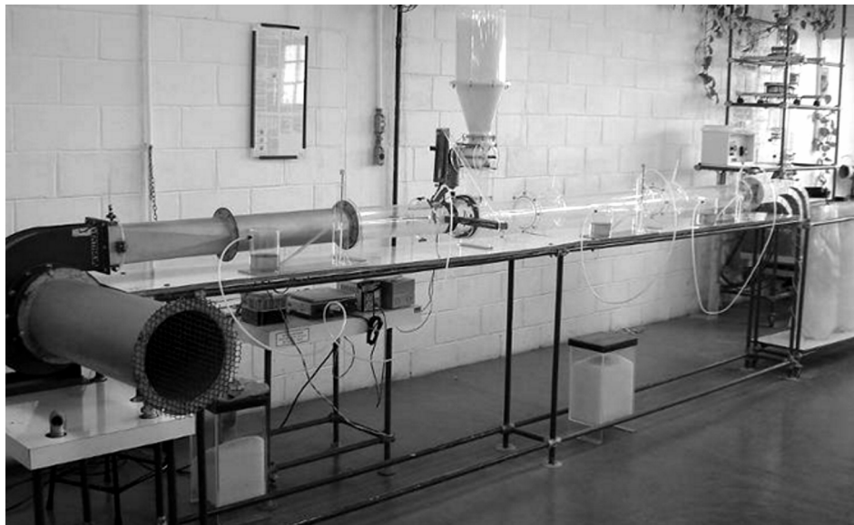
Figure 2: Pilot pneumatic conveying system: installation view.
