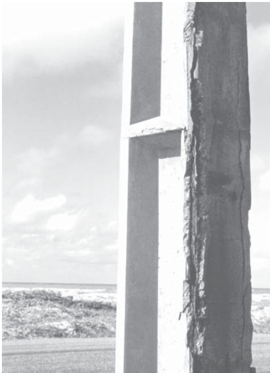
Figure 6: Concrete utility pole presenting chloride corrosion attack, at Aracaju.
