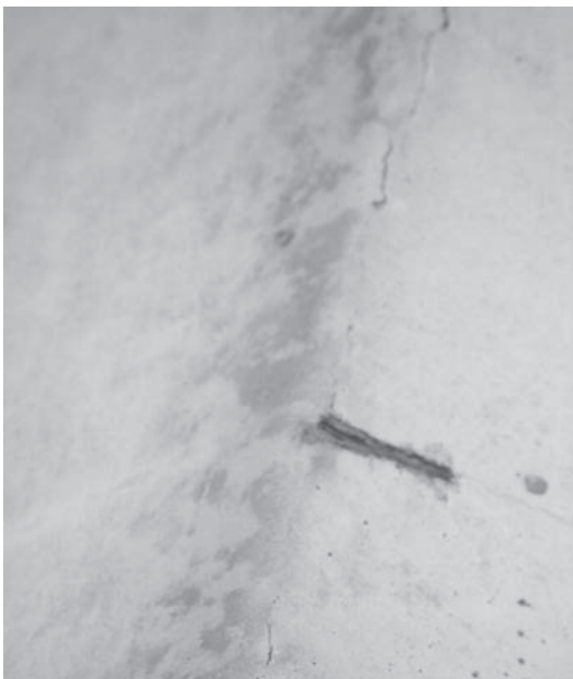
Figure 11: P232 utility pole presenting color alteration on the concrete surface, at rebar direction (iron smudges), superficial cracks and corrosion of steel reinforcement.
