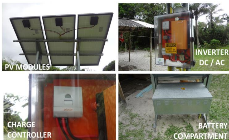
FIGURE 8. Photovoltaic installation details in Cambriú and Foles communities – PEIC-SP. Source: research database, 2014.
