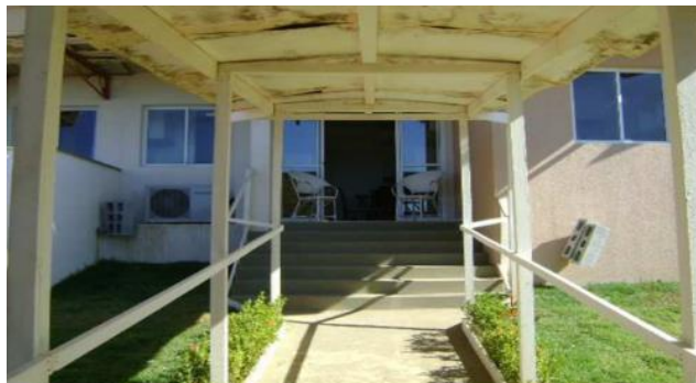
Figure 13. Protected sidewalks and access to the site. Source: the authors.
