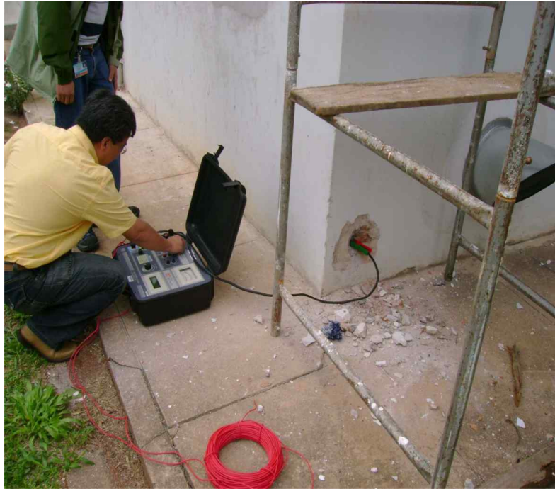
Image 08 - Technicians from the Institute of Electrotechnology and Energy - IEE/USP analyzing the possibilities of deploying a lightning rod system through the building's metal frame. Source: Elaborated by the authors.
