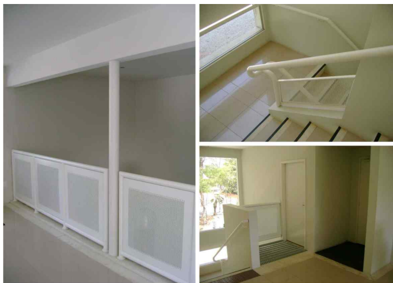
Image 07 - Guard rails installed in Building 19 of CIENTEC. Source: elaborated by the authors.
