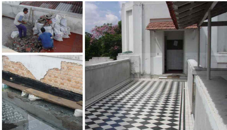
Figure 04 - Full replacement of the slab weatherproofing system for CIENTEC Park's main building (Building 05, Administration). Source: elaborated by the authors.
