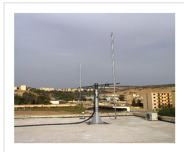
Figure 2. VHF/UHF antenna structure.
