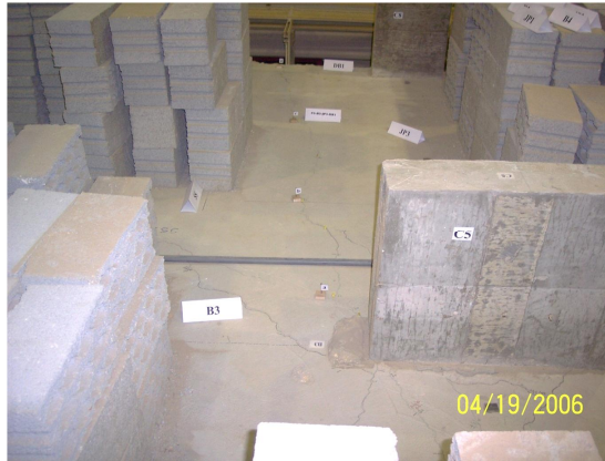
Figure 5 Photographic documentation of crack patterns on C5-C8 path
