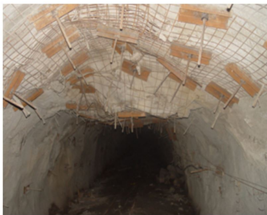
(a) Rheological failure of roof
