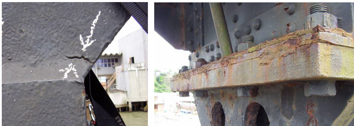
Figure 9: Fissures and the high corrosion level at the pylon base.
