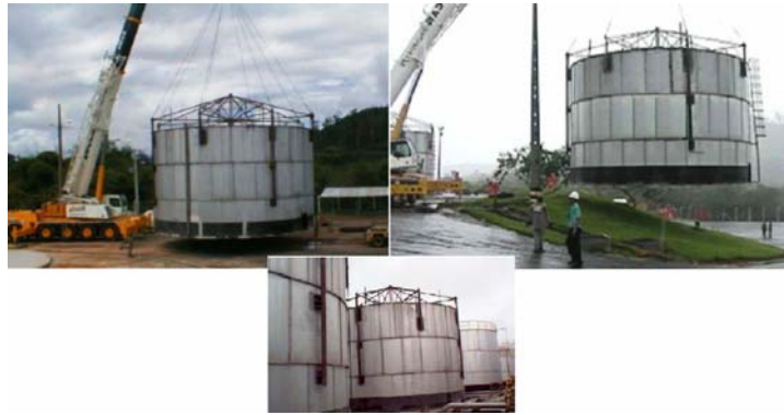
Figure 5: Transport of an ethanol reservoir by a crane using a special truss lifting system attached to the tank through bonded joints.
