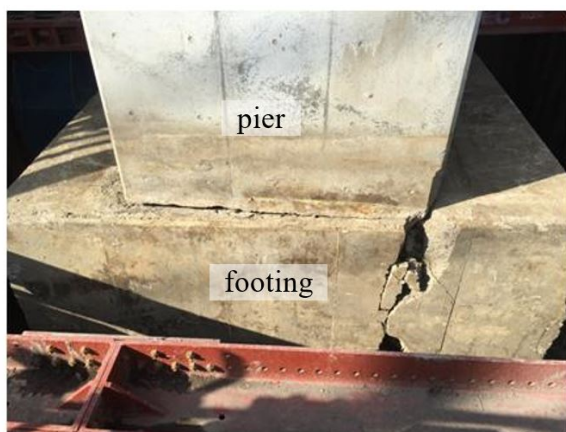
(a) earthquake-induced footing damage
