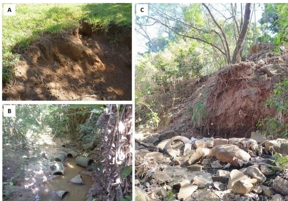
Figure 5 - [A] Riverbank erosion caused by runoff drained into the permanent preservation area of Buritizinho Stream, Uberlândia - MG. [B] Perpétua Stream silted bed, Uberlândia-MG. [C] Riverbank erosion in the Buritizinho Stream, in the image it is possible to identify that the erosion process is already beginning to compromise the stability of the existing vegetation in the place, exposing the roots of the trees
