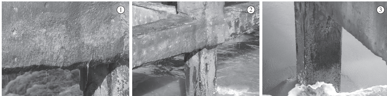
Figure 1, 2 and 3. Growth of marine seaweed on structural components.
