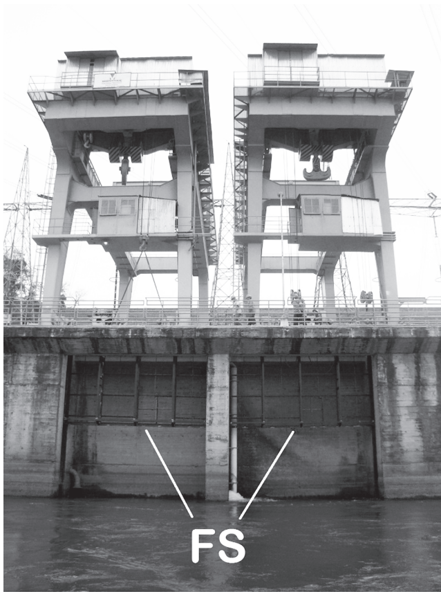
Fig. 2. Fish screens (FS) used to block the entrance of mandi into the draft tube of Três Marias Dam during turbine stop/startup.
