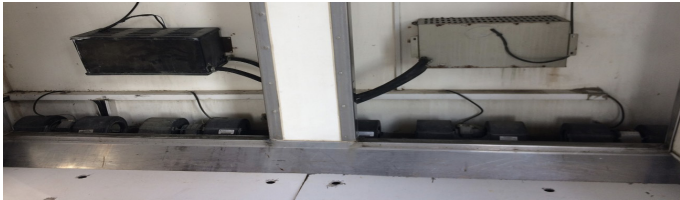
Figure 2 – Mechanical ventilation engines.
