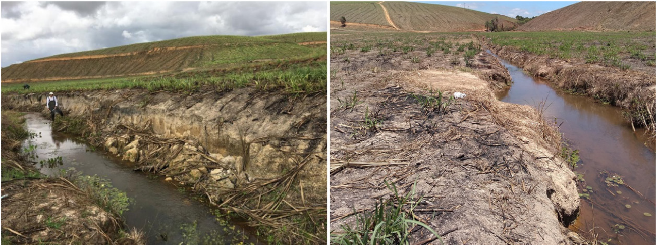
Figure 7. Channel banks evidencing collapse or exposed without riparian vegetation in the middle course of the Sapocaji sub-catchment.
