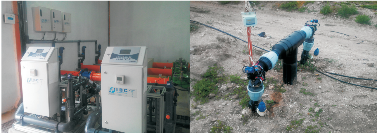
Figure 2 - Irrigation control equipment, programmer and solenoid valve.
