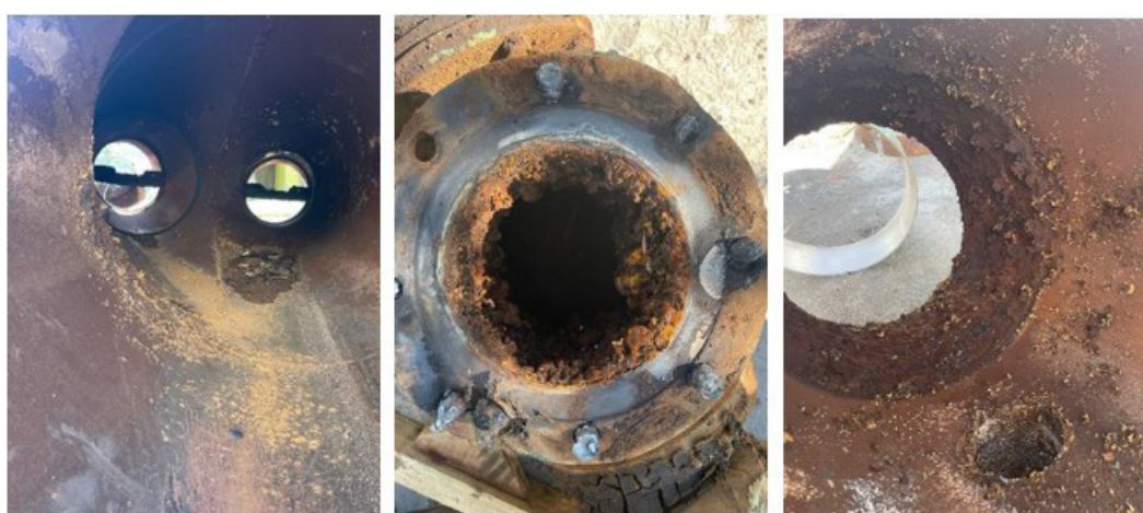
Figure 3. Detachment material in pipeline.
