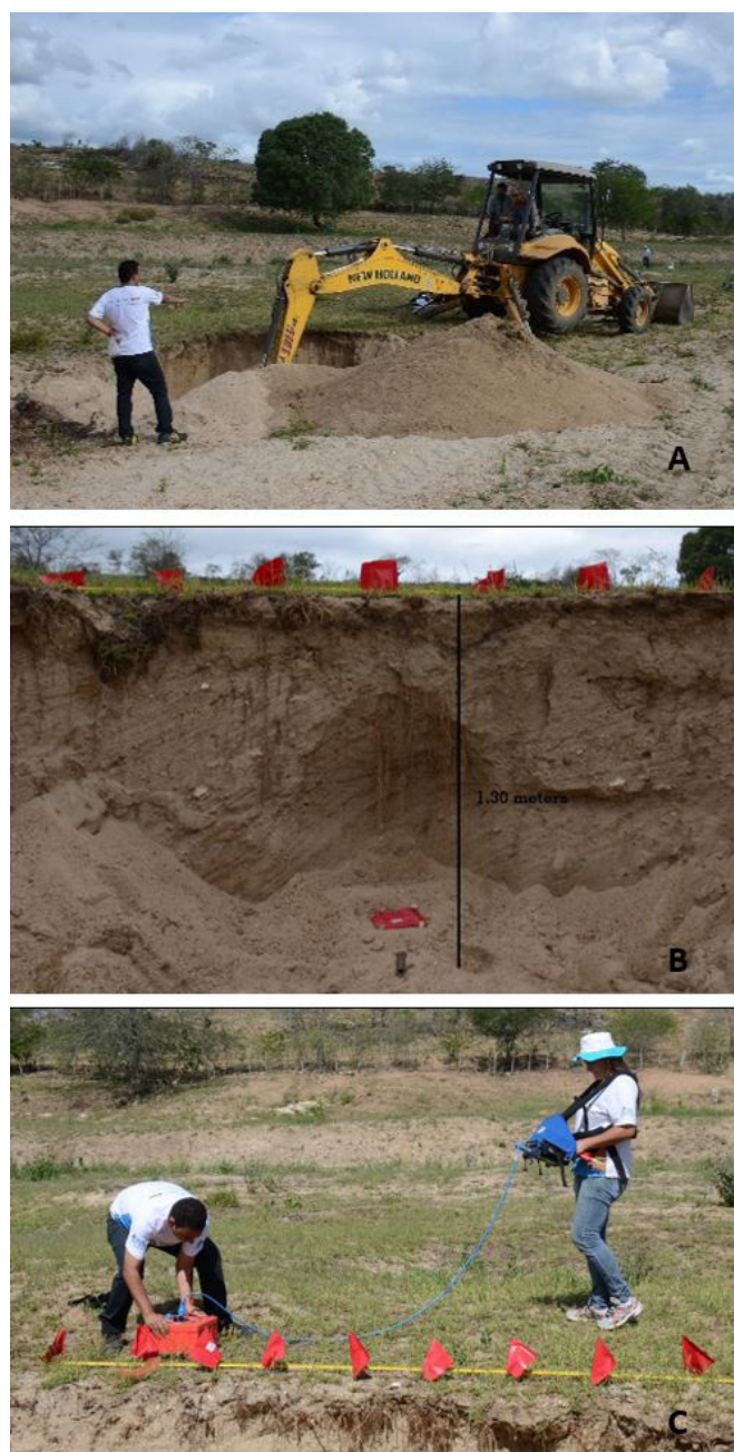
Figure 4. Secondary trench in the Upper Capibaribe River, Case 2. (A) Construction of the trench; (B) Position of flags and the iron bar and (C) Application with antennas of 400MHz e and 200MHz parallel to the cut made on the slope antenna.
