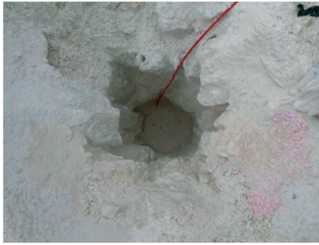
Figure 6 Cracked hole collar and hardened plaster
