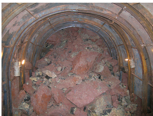
Figure 1 - Collapse during drilling in a water gallery in the Canary Islands.
