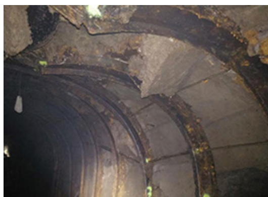
Figure 2 - Overloaded arch in gallery section.
