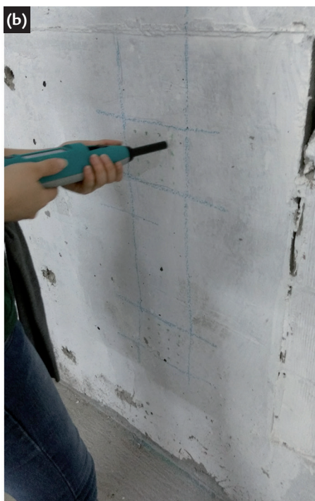
Figure 3 Surface hardness test: (a) marking the points with the test gauge (b) placement of the Schmidt hammer.
