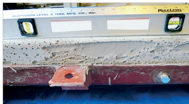
Figure 11 Discontinuities on the concrete core
