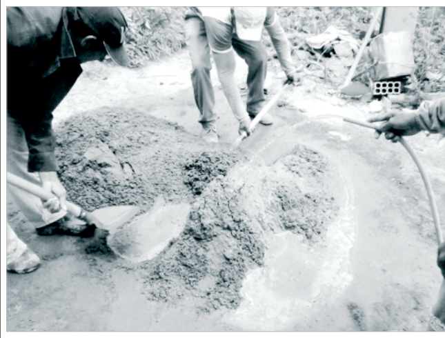
Figure 7 – Incorrect addition of water to the concrete
