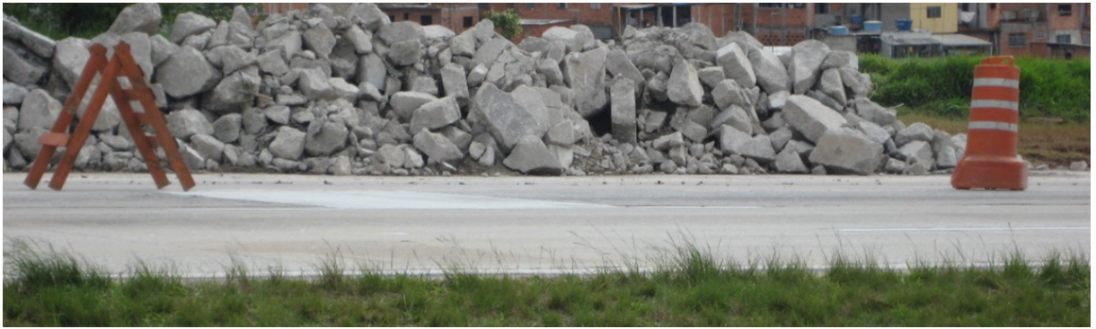
Figure 4. Broken-up concrete slabs collected from right lane at KM 24 km.
