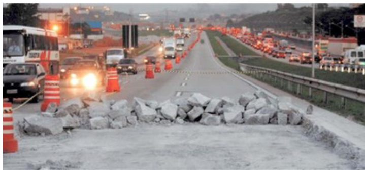
Figure 1. Slabs removal at left lanes at kilometer post (KM) 22 in 2003. (Reproduction: Folha de São Paulo newspaper).
