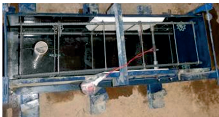
(b) Formwork for casting of column of model with corbel cast in different stage
