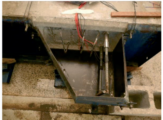
(b) Main and loop reinforcements of corbel ready to be cast (model P2)
