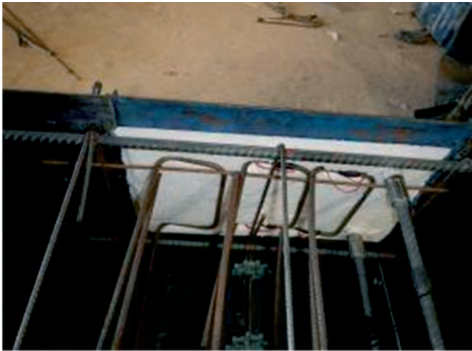
(a) Placing of Styrofoam plate for creating shear key and detail of loop reinforcement bent on formworks before casting of the column (model P2)
