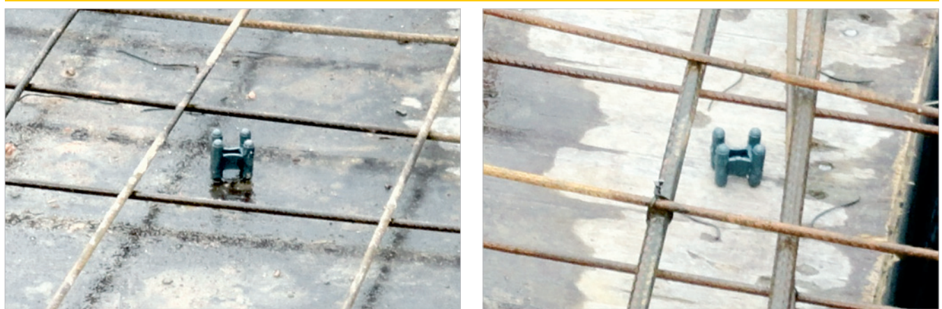
Figure 4 – Spacers that came loose from the reinforcement, no longer performing its function
