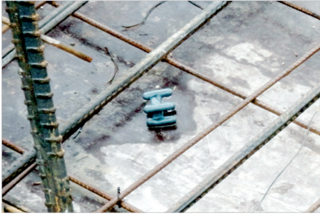
Figure 5 – Spacer that tumbled during a concreting operation
