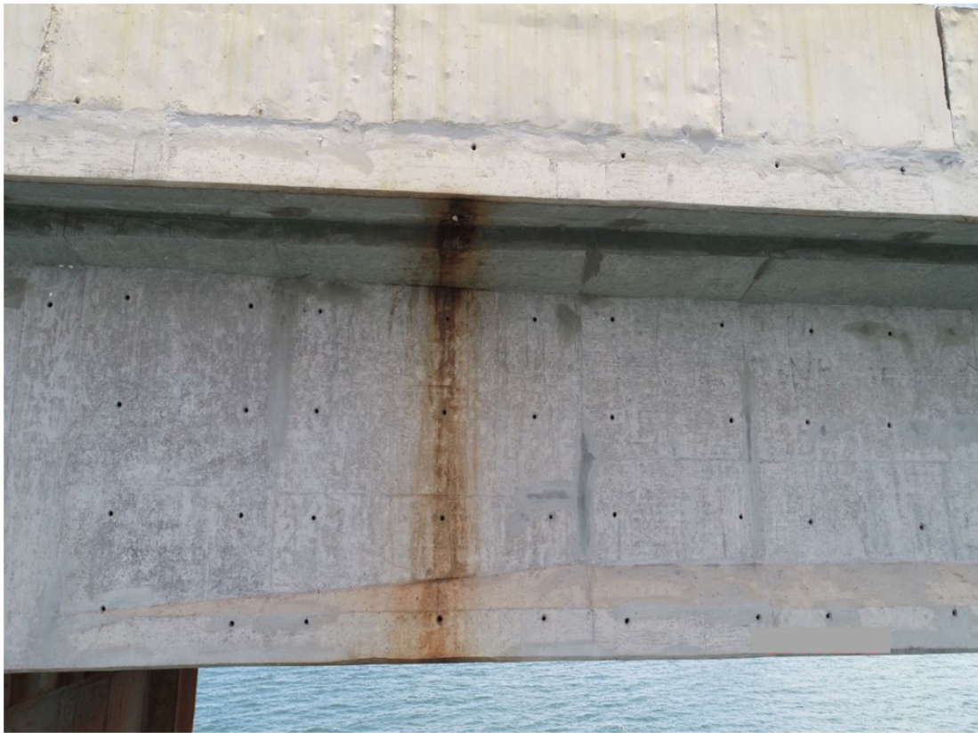
Figure 10. Span 12 of the longitudinal beam 2, with signs of water infiltration. It was possible to note the absence of an extension tube on the drainpipe.
