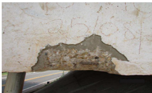
a) Longitudinal beam 3, on overhang 3, with crumbling concrete and exposed reinforcement
