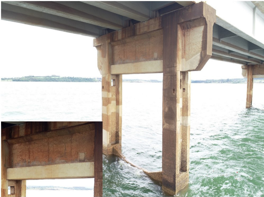
Figure 8. Crossbeam 11 with cracks
