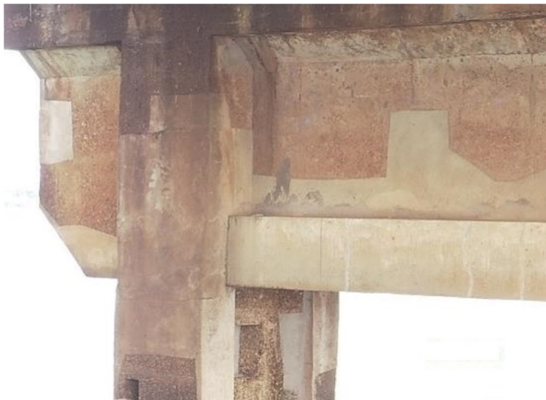
Figure 9. Pillar of support 21 with cracks on the repair.
