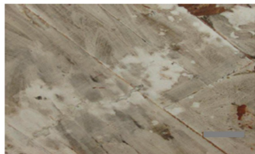
b) Deck slab with crack showing efflorescence
