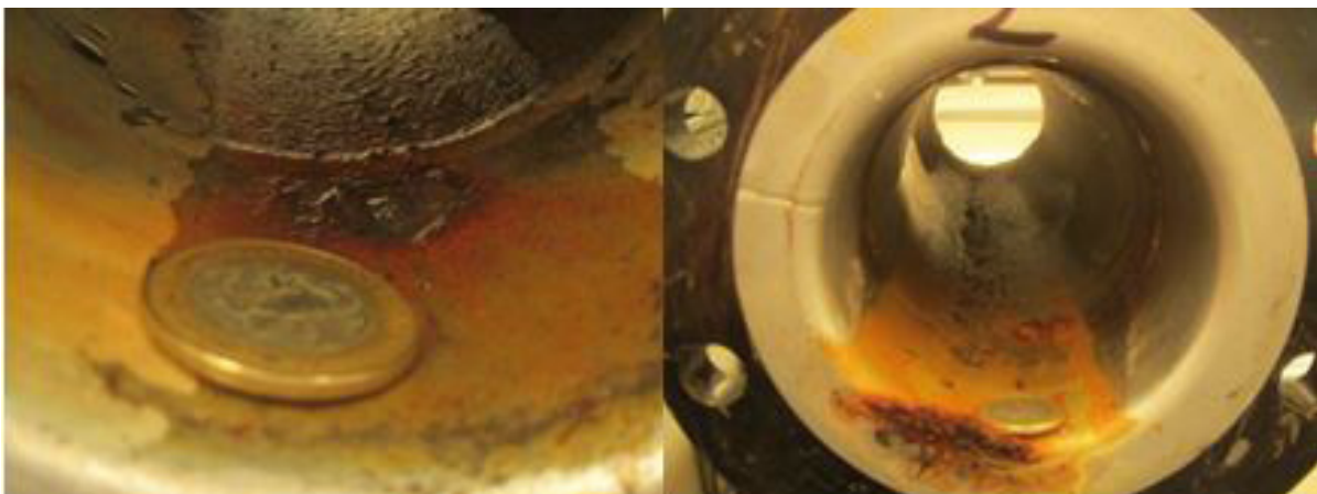
Figure 1. Damaged tubes of chiller under analysis. It is seen evidence of reddish corrosion products.
